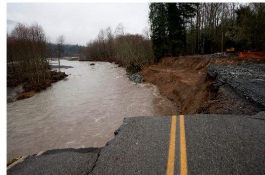
North Fork Road after being washed away by the Nooksack River. December 2021, Bellingham Herald
