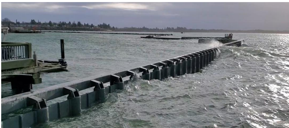
King tide at Blaine Harbor wave wall, December 2022
