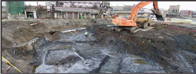
The Port has partnered with the Department of Ecology to clean up historic contamination and prepare the Waterfront District for redevelopment
