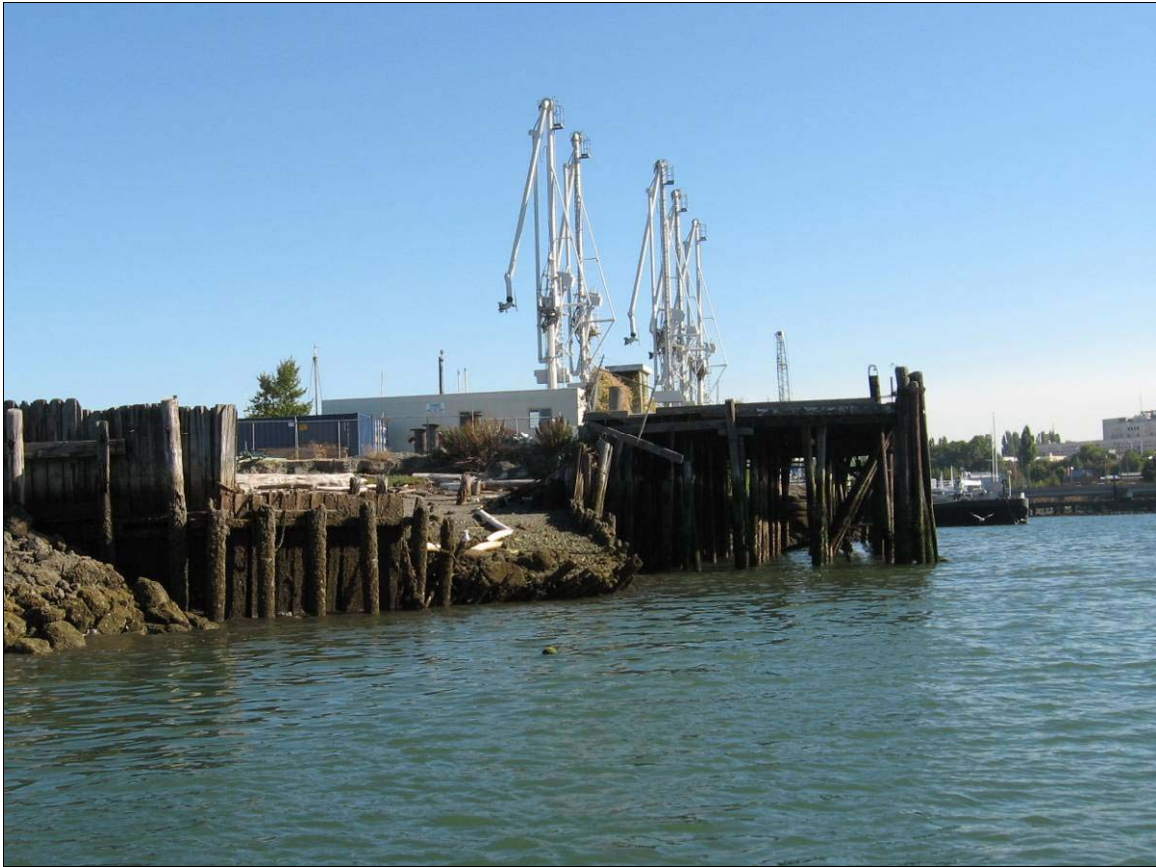
Photograph 3. Failing bulkhead, overwater piers in Area 1
