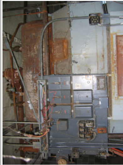
View of Mechanical Equipment taken 8/29/2006 Photography Neg. No (Roll No./Frame No.): 12 Comments:
