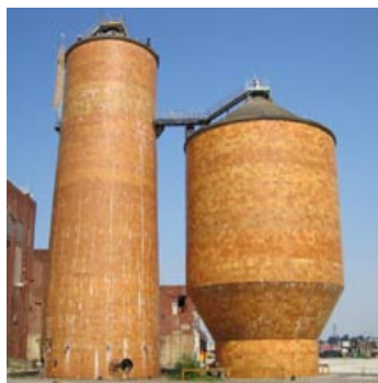
#49 High Density Tanks
